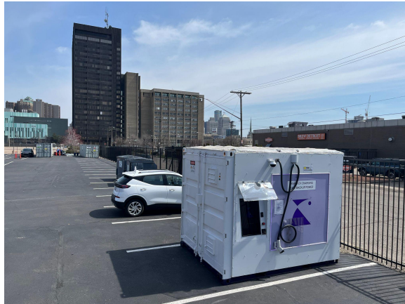
Figure 2: ElectricFish unit deployed at IBEW Local 58's Zero Net Energy Center with Stargazer™
